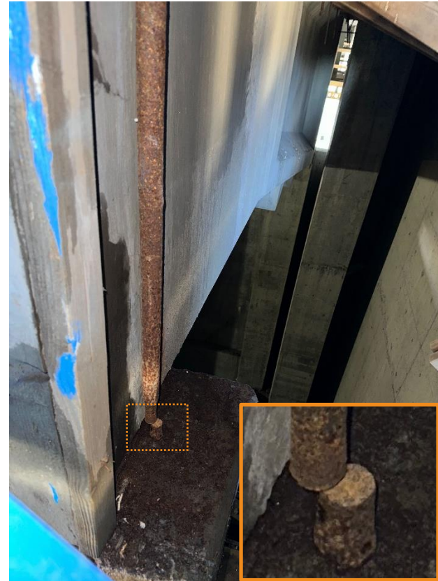
Figure 2. Pier 7 Cantilever F fractured tie-down rod
